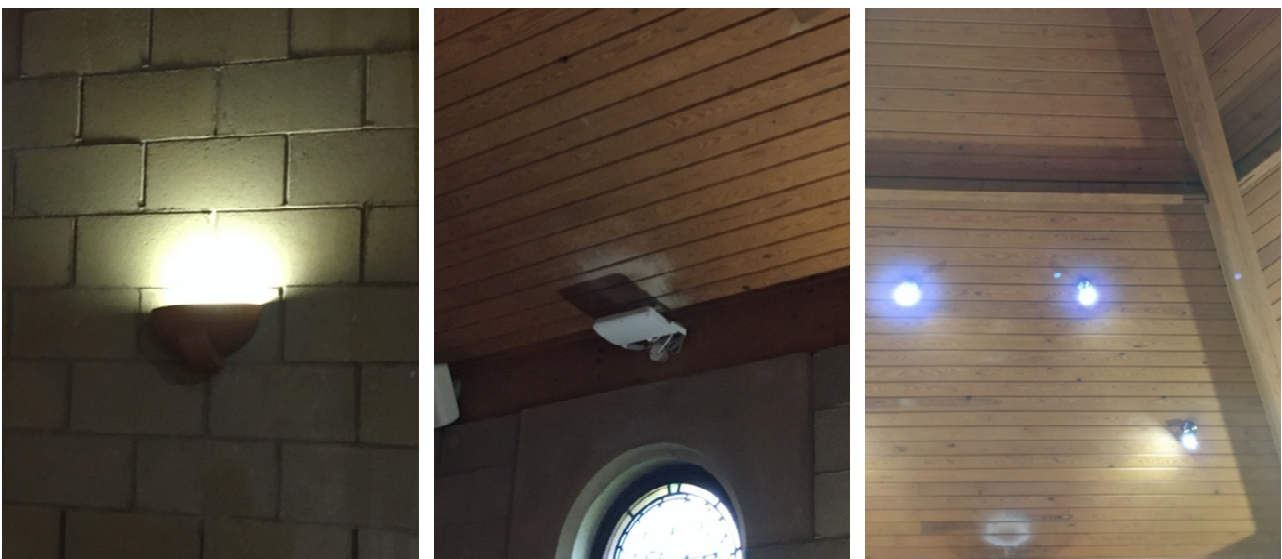
Photographs 7, 8 & 9: Church Light Fittings
